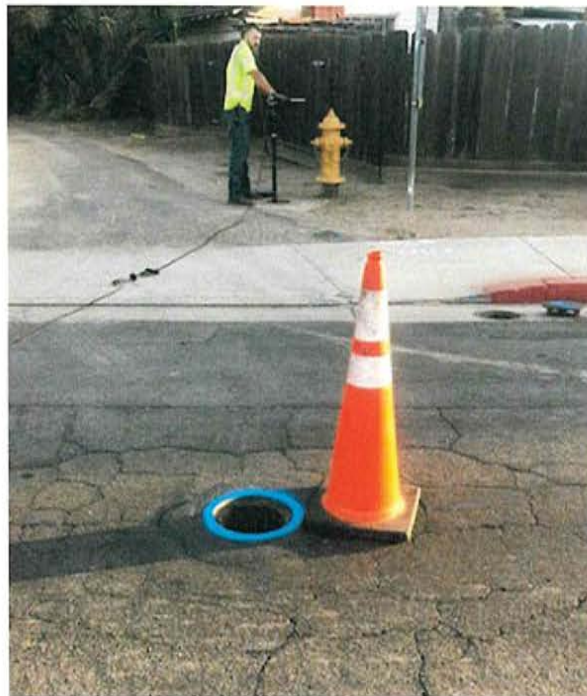
Figure 3.1: Valve Lid Cover Missing
